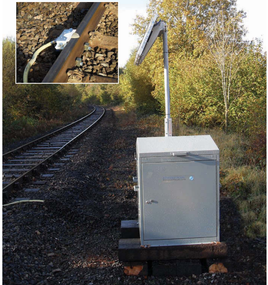
Portec's spreader bar (inset) places a compact layer of traction gel on the rail head, supplied from a trackside cabinet..
